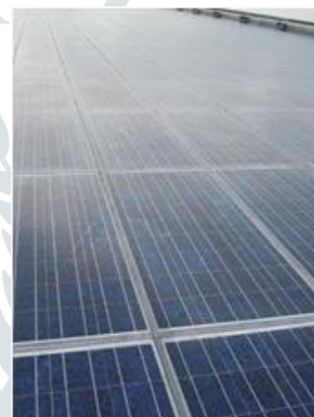
Polycrystalline modules (47.28kWp) on the main roof
