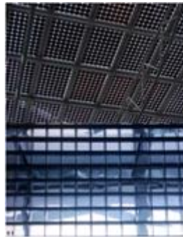
Glass semi-transparent PV modules (11.64kWp)
