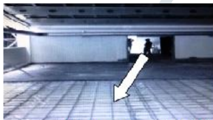
Polystyrene layer is installed on the uppermost floor of the office building (Source: Malaysia Green Technology Corporation, 2010)
